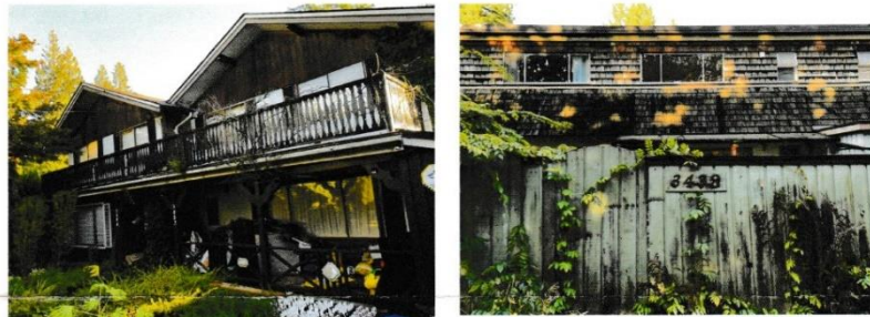
Above: The existing structures have been deemed hazardous by Spratt Emanuel Engineering Ltd. and face serious challenges including mold, leaks and structural problems.
